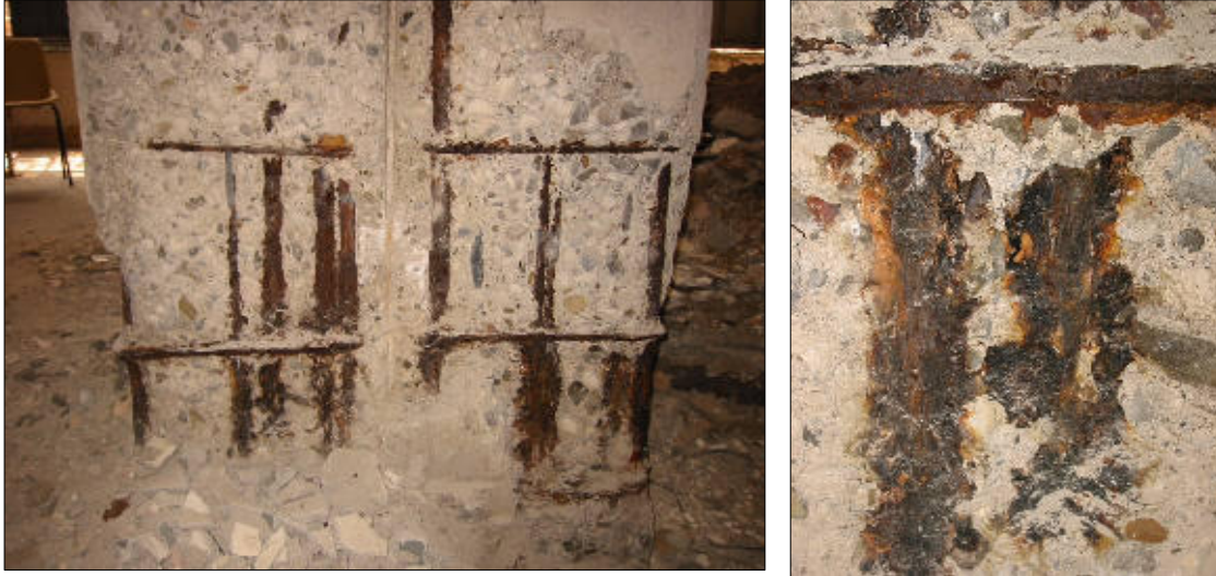
Fig. 6. Corrosion of the steel reinforcement at the bottom of the columns, sector B3
